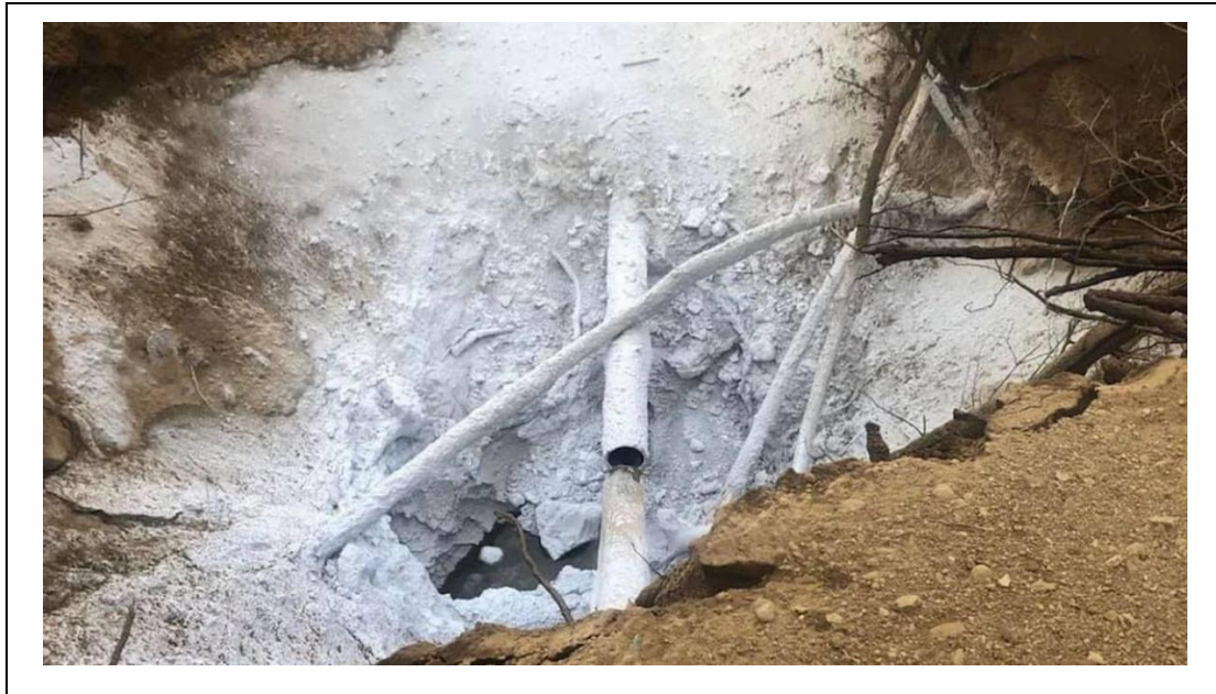
Figure 5: Close up photograph of a CO 2 leakage from the rupture of a Denbury Resources CO 2 pipeline in Yazoo County Mississippi, USA 22 February 2020 showing to localise freezing caused by the Joule Thompson effect
